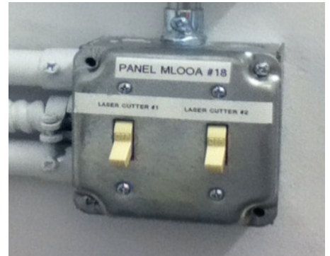
Figure 1: Laser Cutter and Fan Exhaust Power Switch
