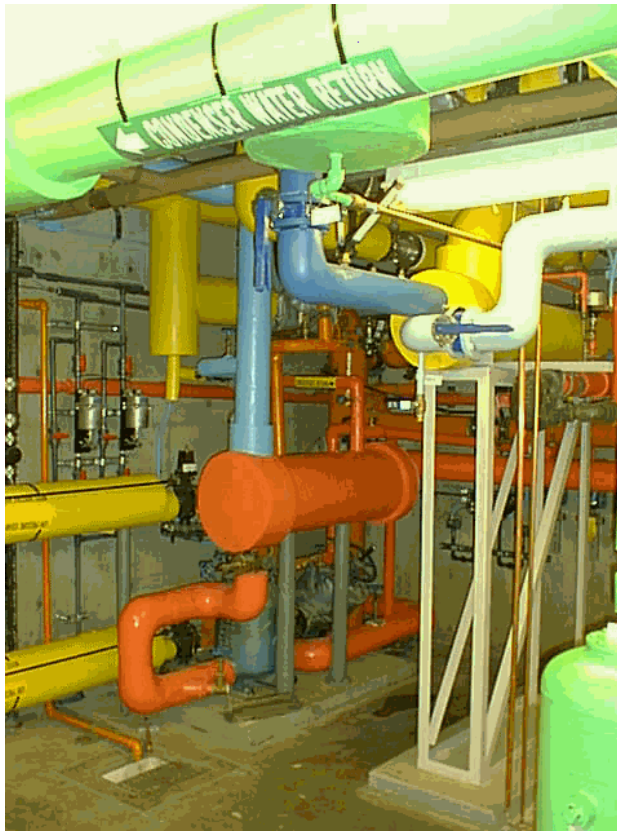
Figure 3. The machine room is color-coded and visible behind a glass wall.
